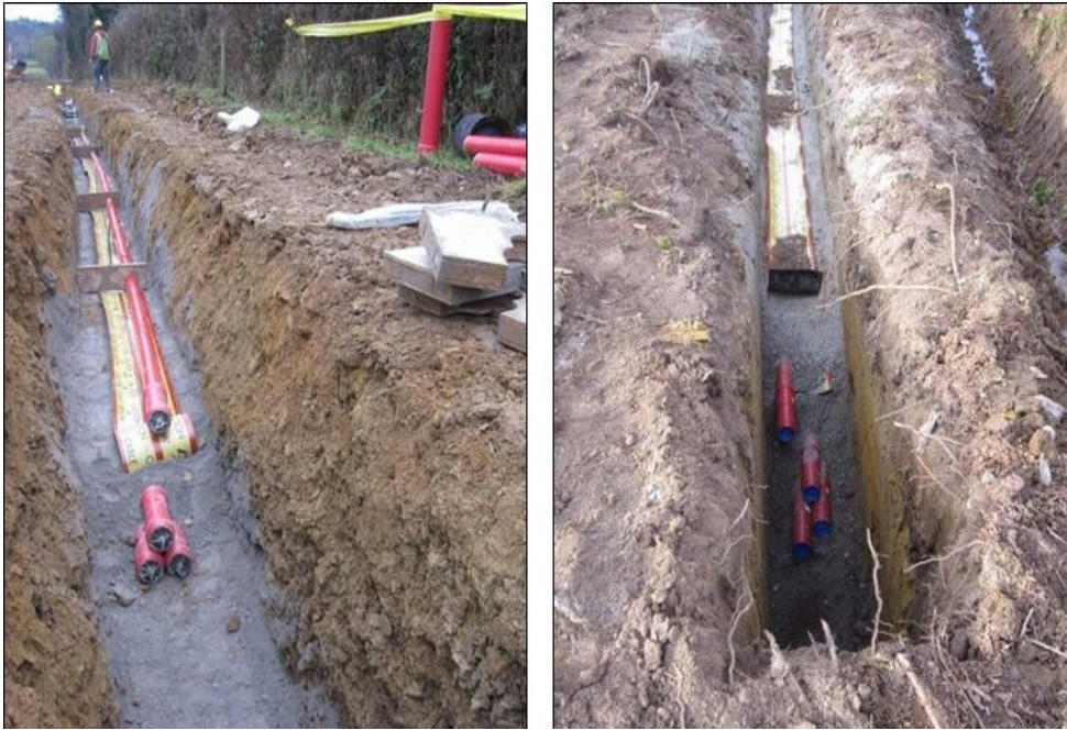
Plate 4-8 Typical Cable Trench View
